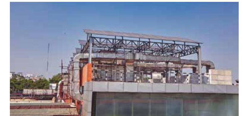
Solar plant installed to reduce electricity consumption.
