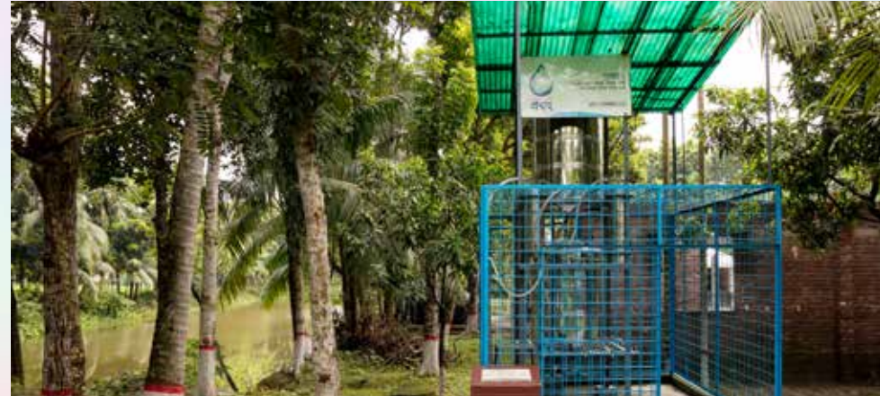
Water filtration plant at Manikgonj
