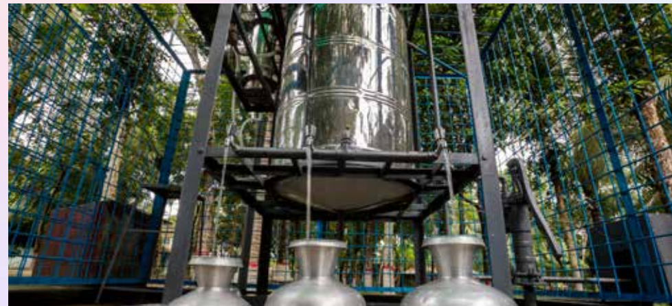
Water filtration plant at Kushtia
