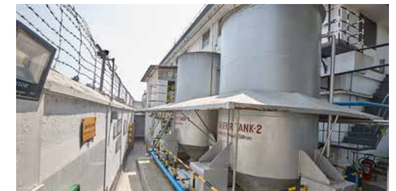
ETP inside the factory.
